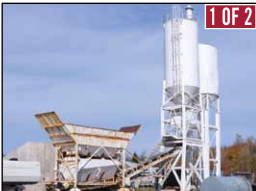
(2) Cement Batch Plants
