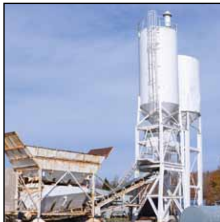
Large Cement Plant
