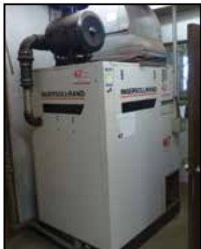
INGERSOLL-RAND 50-HP Air Compressor
